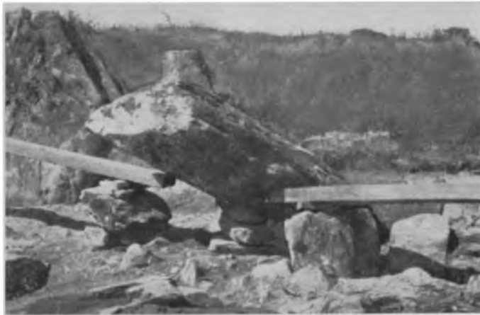
(a) Re-erection of stone no. 16. Note wooden pegs beneath the levers and packing stones underpinning the slab
