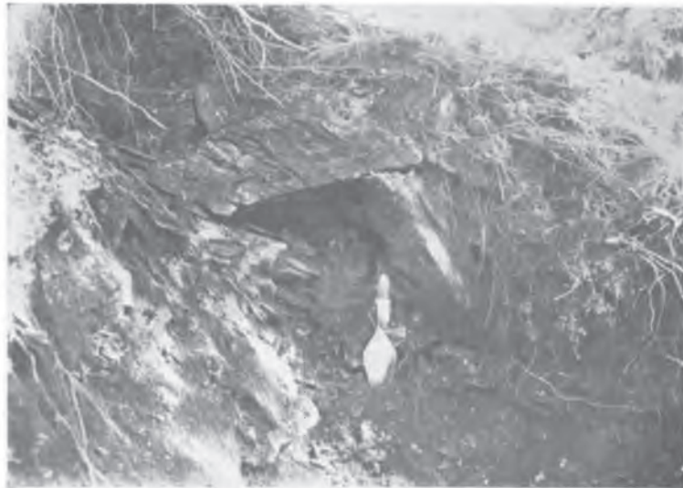
Showing evidence of slip of material from inside the retaining wall
